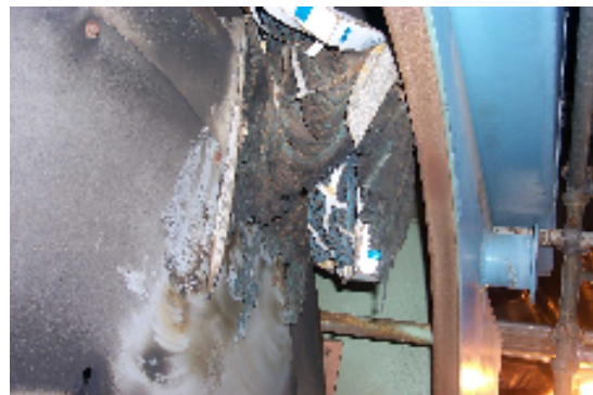
Figure 4: Dirty paper filter was sucked into motor
