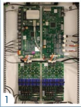
1 MAINS CONTROL ASSEMBLY
